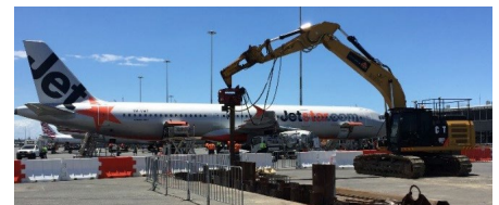
JOINT USER HYDRANT INFRASTRUCTURE TIMING: 2017 - 2018 | VALUE: $6.3M
