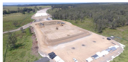
PACIFIC HIGHWAY UPGRADE WOOLGOOLGA TO BALLINA WAVE 4 EARLY WORKS TIMING: 2016 - 2017 | VALUE: $49M
