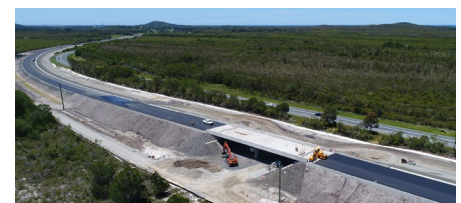
PACIFIC HIGHWAY UPGRADE W2B WOODBURN TO BROADWATER SERVICE ROAD TIMING: 2017 - 2018 | VALUE: $41M
